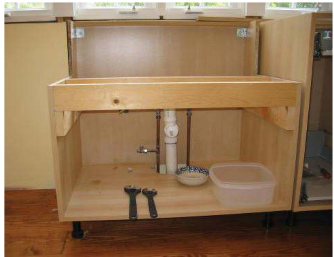
[Above]: The cabinet is now fully installed, and ready for the sink to be set in.
