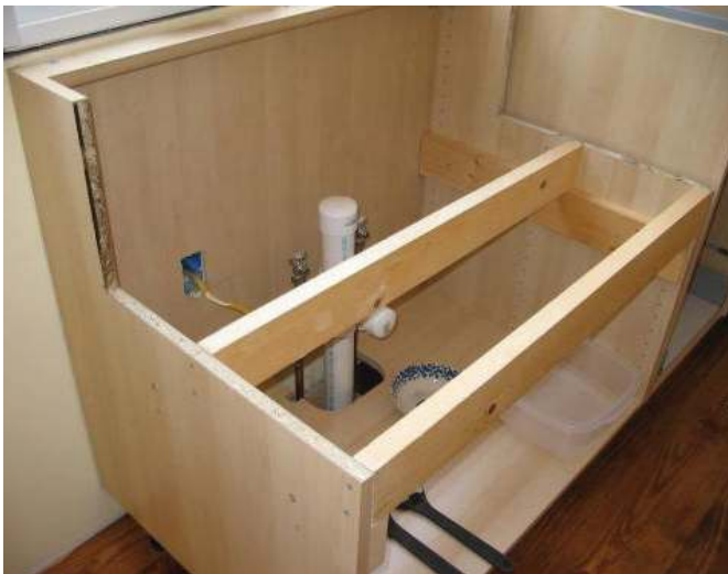
[Above]: The cabinet is lifted up over the plumbing, and set in place
